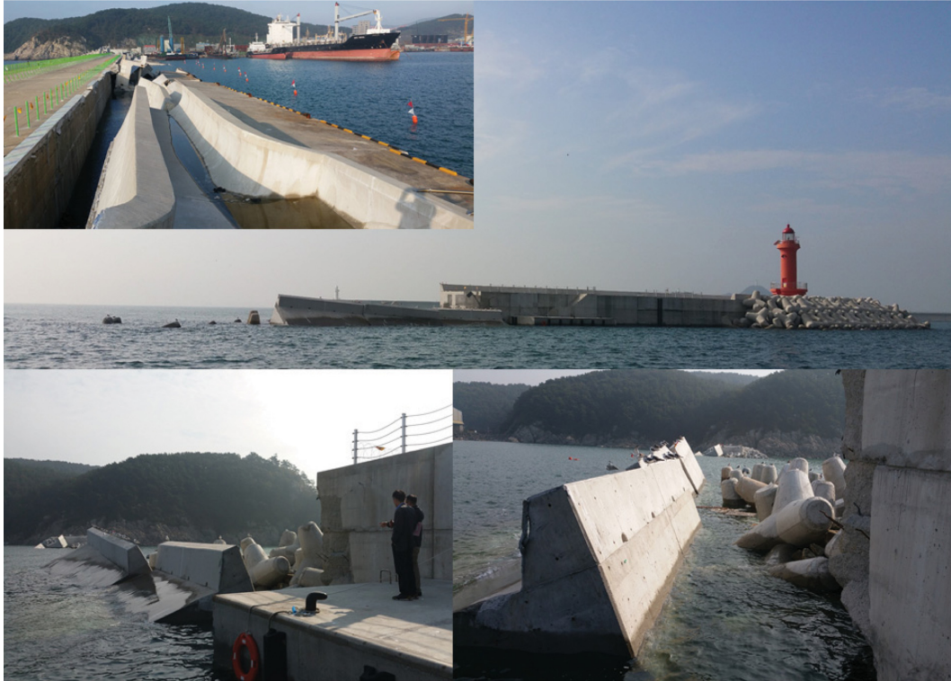
Fig. 2. Breakwaters destroyed by Typhoon CHABA.
